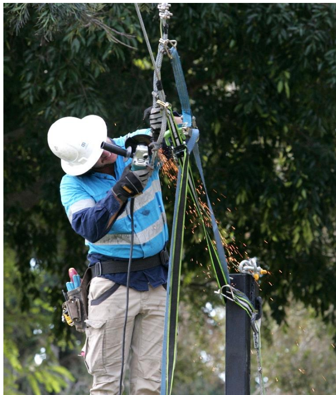
Above and below: Telco Antennas inspecting, repairing/replacing and optimising antennas, connections, cabling and fittings on our radio mast.
